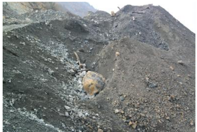
Figure 4: View of a sinkhole that emerged in the Southern area
