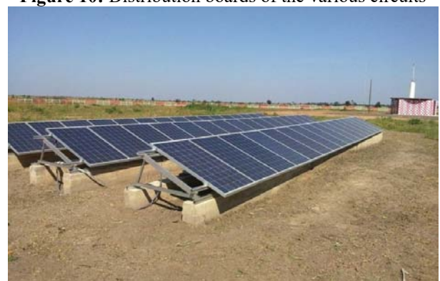
Figure 11: The photovoltaic system and the VOR station.
