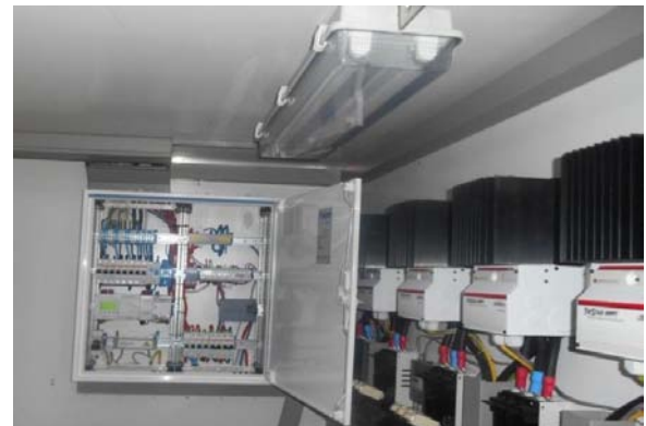
Figure 10: Distribution boards of the various circuits
