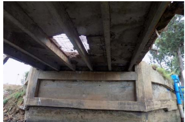
Figure 14: Falling off of the plastered underside of the superstructure slab aimed at concealing the reinforcement bars
