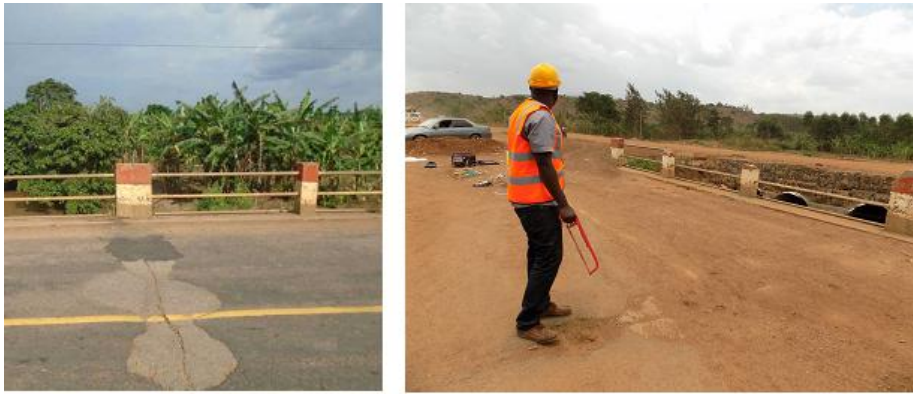
Figure 15: Transverse crack in the slab running to the bottom of the layer
