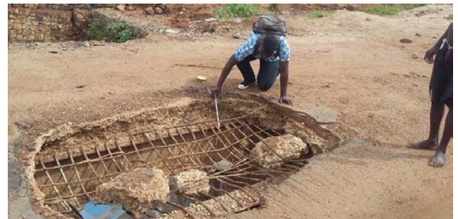
Figure 12: Bottom reinforcement at failed slab location. The reinforcement is diameter 16mm round bars at 100mm centres
