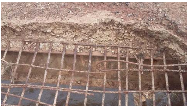
Figure 2: No hogging reinforcement in the slab, the concrete looks generally weak with a higher percentage of coarse materials
