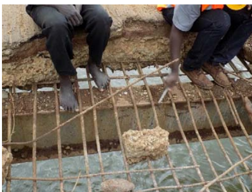
Figure 3: The longitudinal steel beams appear to have no shear connectors
