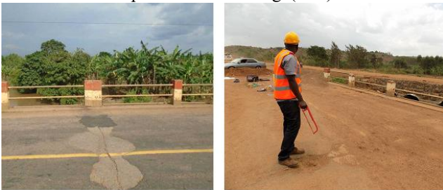
Figure 8: Transverse crack in deck surfacing and concrete patching. There is no transverse joint in the concrete slab on the underside
