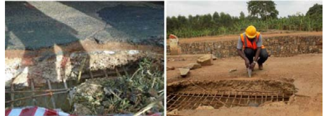
Figure 11: Opening in superstructure slab showing longitudinal steel beam, bottom reinforcement, disintegrated concrete layer and gravel layer under surfacing. No hogging reinforcement over longitudinal beams
