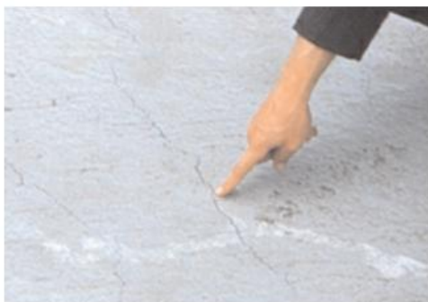
Figure 7: Typical plastic shrinkage cracks
