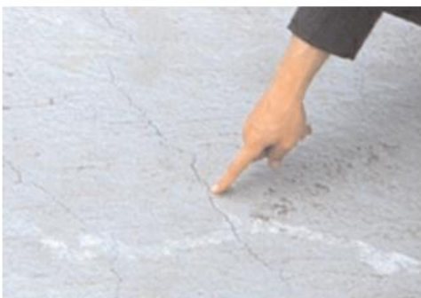
Figure 7: Typical plastic shrinkage cracks
