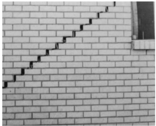
Figure 2: Typical severe diagonal deep crack in the wall
