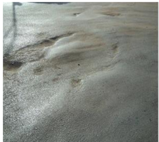
Figure 3: Severe distresses of heave on Alarda road, [13]
