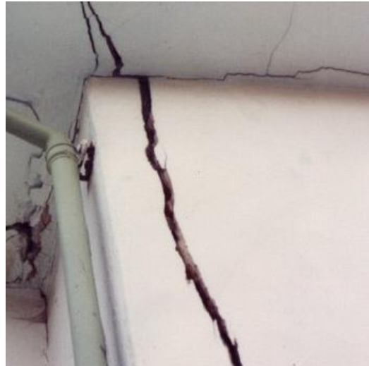
Figure 5: Severe wide cracks in walls and roof
