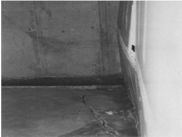
Figure 4: A severe cracks of ground floor and inside walls
