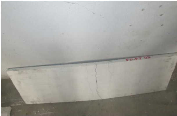
Figure 12: (b) Crack Pattern (FP- FT02)
