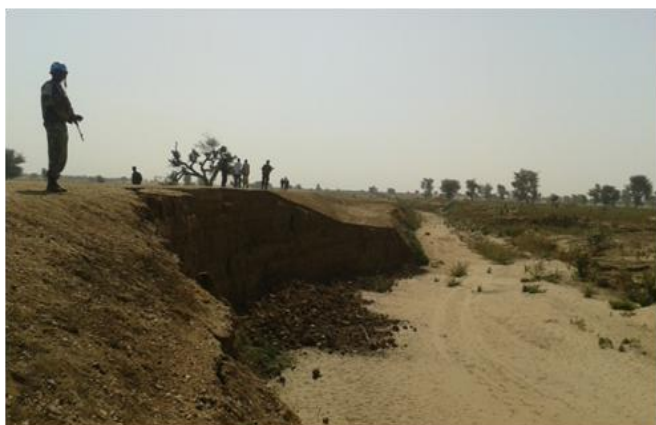
Figure 4: Weak and steep slope of the embankment
