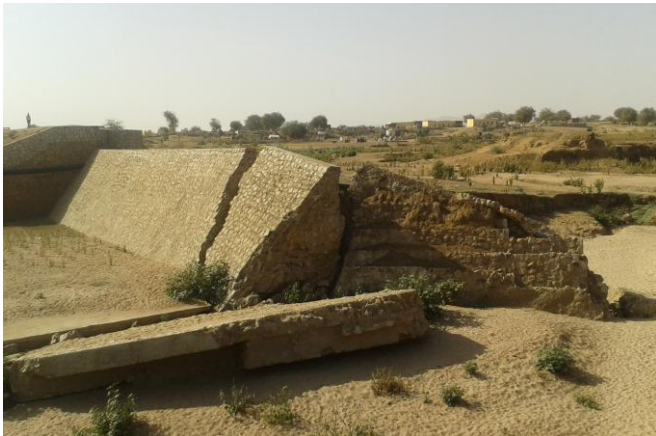
Figure 3: Damaged spillway with severe cracks
