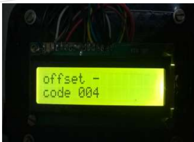
Figure 6(b): LED display showing Offset Misalignment
