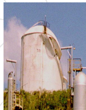
a) Elephant-foot buckling b) Damage to the roof or the Upper shell of the tank
