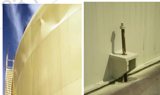
c) Sloshing damage to the shell of the tank d) Inelastic stretching of an upper shell anchor bolt at the tank base
