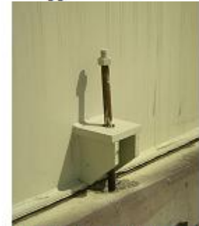
d) Inelastic stretching of an anchor bolt at the tank base
