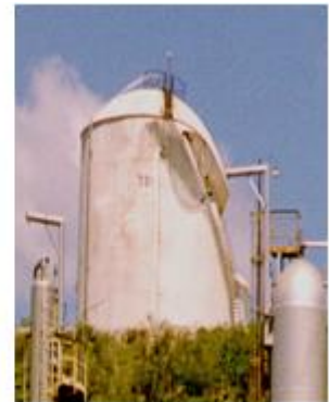
b) Damage to the roof or the Upper shell of the tank
