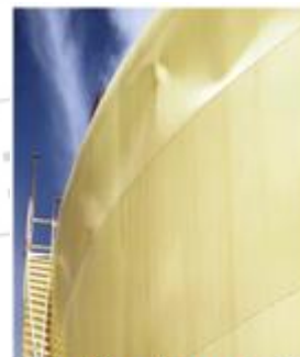
c) Sloshing damage to the upper shell of the tank
