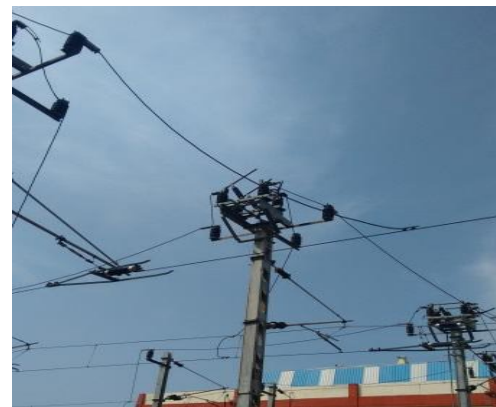
Figure 1: Overhead line for traction
