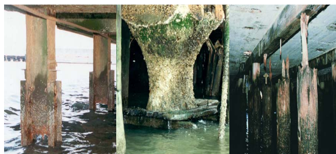
(a) (b) (c) Figure 1 Degradation of conventional marine piles (a) Corroded steel piles b) Degraded concrete pile (c) Deteriorated timber piles, [2].
