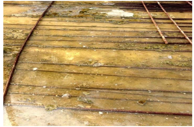
Figure 6: Rebars Placed Get Exposed to Water, Resulting in Rusting
