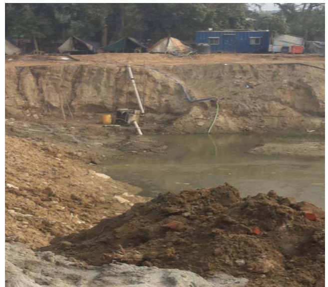
Figure 3: Muck And Stagnated Water, Unworkable Conditions Due To Improper Dewatering.
