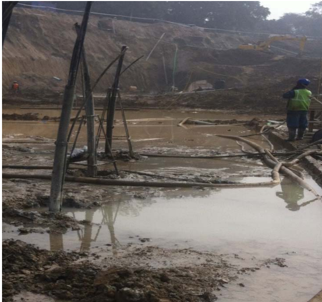
Figure 7: Deposition of Muck Due To Ruptured PCC
