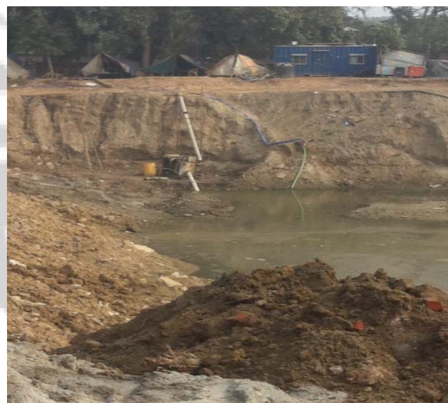
Figure 3: Muck And Stagnated Water, Unworkable Conditions Due To Improper Dewatering.
