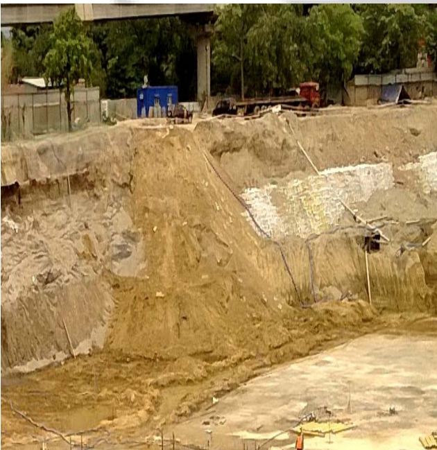
Figure 5: Soil Erosion From Earth Brim Due to Delay in Shotcrete.
