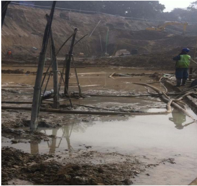
Figure 7: Deposition of Muck Due To Ruptured PCC
