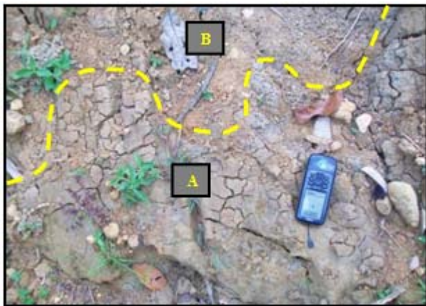
Figure 7: Claystone (A) mixed with landslide material (B) that comes from top of the slopes
