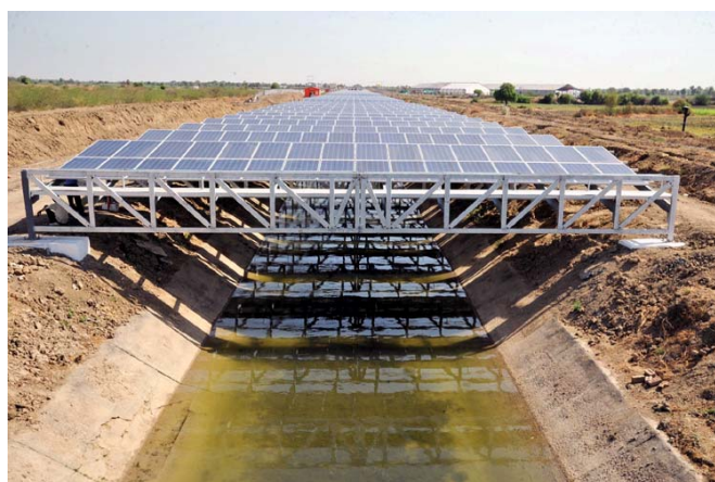
Figure 1: India's 1 st 1 MW Canal-top solar power project in Gujarat
