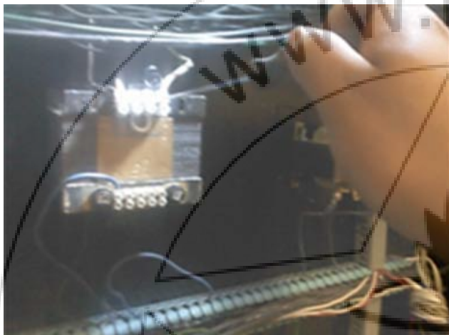
Figure 4: 440/127 VCA gear Transformers VCA and 440/24
