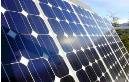
Figure 2: Photo Voltaic Array
