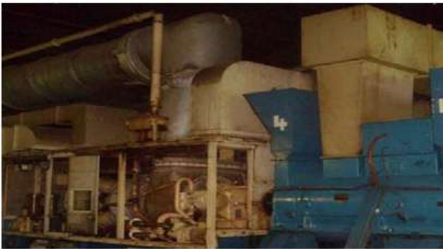
Figure 2: Gas generator-Alternator assembly
