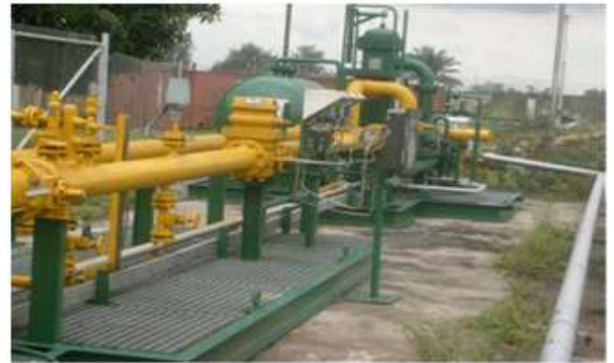
Figure 3: Natural Gas (fuel) Lines
