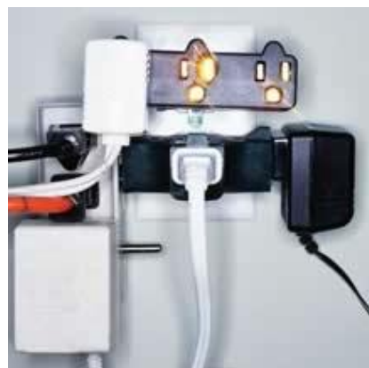
Figure 1: Improper use of an electrical outlet
