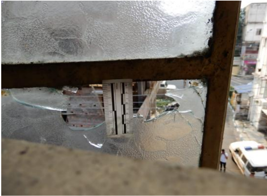
Figure 2: Glass penetration initially reported as bullet impact.
