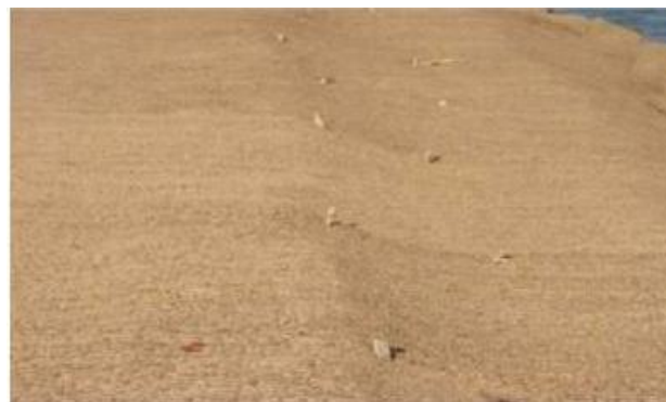
Bamboo pegs inserted to keep the Geotextile in position Figure 8 (a): Field implementation of coir Geotextile
