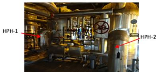
Figure 3.2: High Pressure heater (HPH) PLTU Teluk Sirih Unit 2
