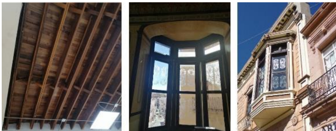
Figure 19: Interior view of the wooden roofs structure, Petit Escobedo's house. Photographer: IRGO, city of Zacatecas, October 21, 2021.
