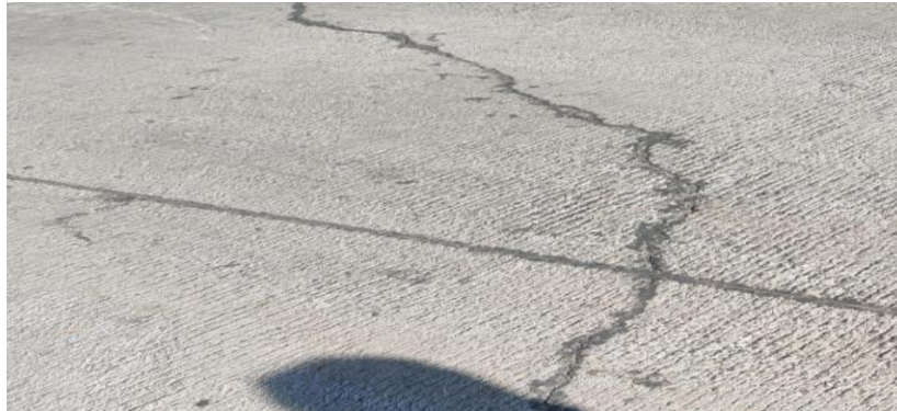
Figure 1: Spalling on Pavement
