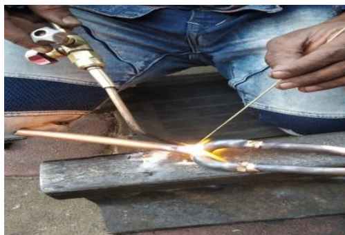
Plate 6: End Pipe Connection
