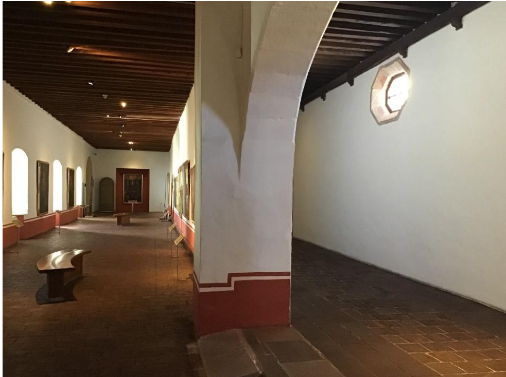
Figure 5: The image allows us to appreciate the thickness of the convent walls Source: IRGO, September 2022.
