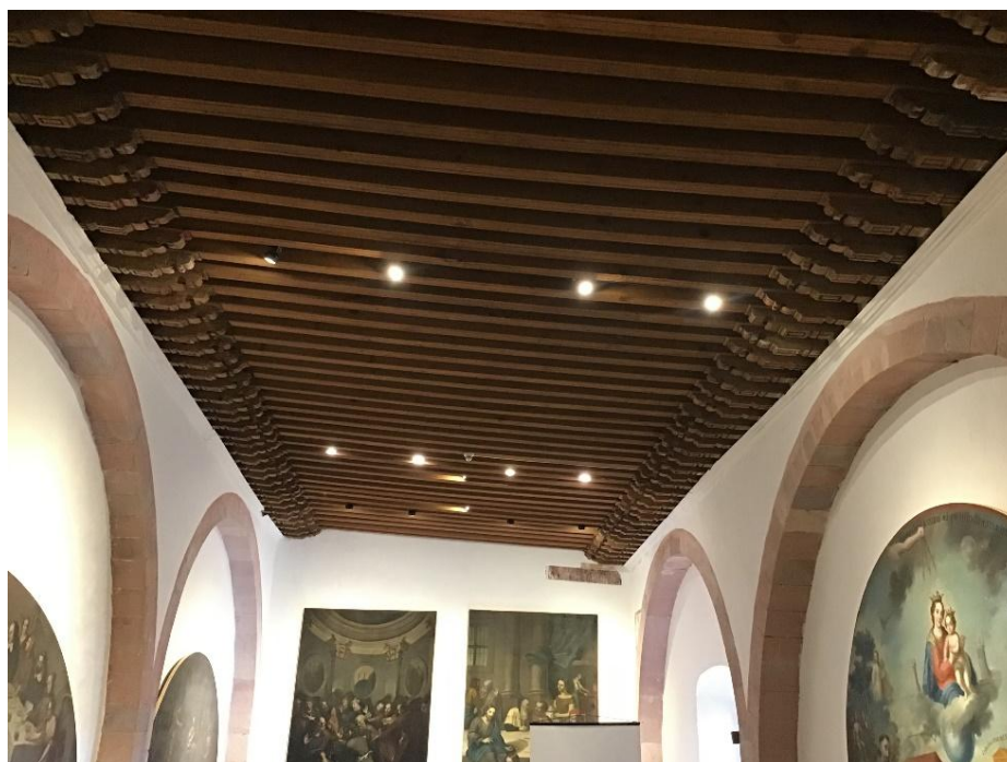
Figure 7: Interior view of another type of beam that formed part of the ceilings of the convent complex. Source: IRGO, September 2022
