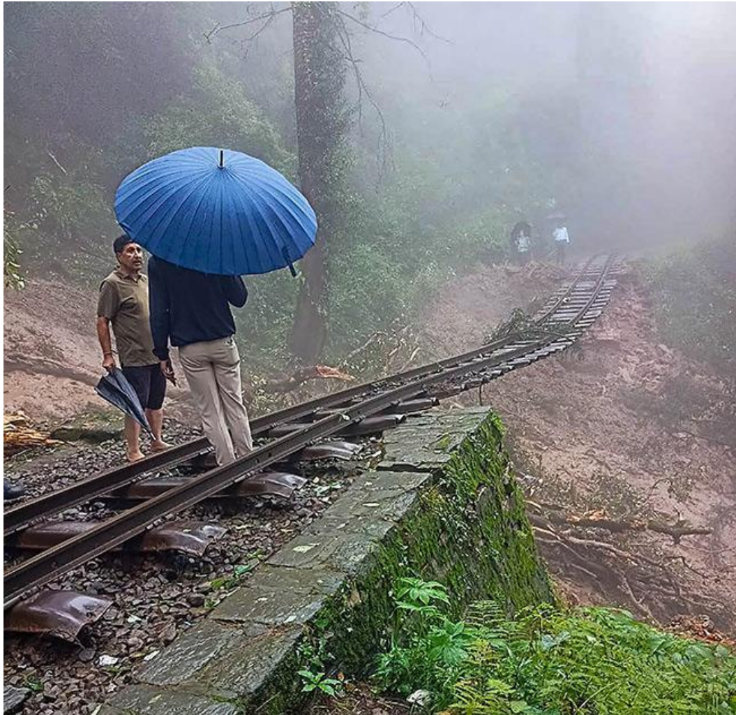
Kalka - Shimla rail track damaged due to land slide.
