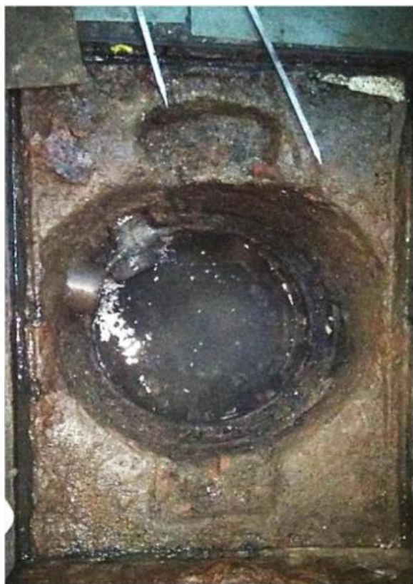
Figure 2: Trial Location 1 - Manhole 1 after 2 weeks application of Biological Solution
