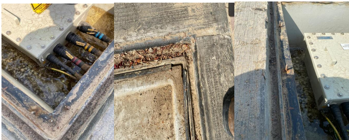
Figure 5: Flush type link box manhole
