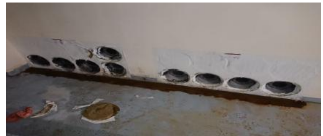
Figure 4: Basement cable entry ducts
