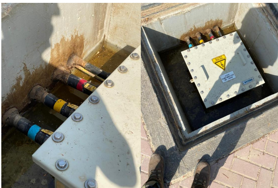
Figure 6: Flush type link box manhole
