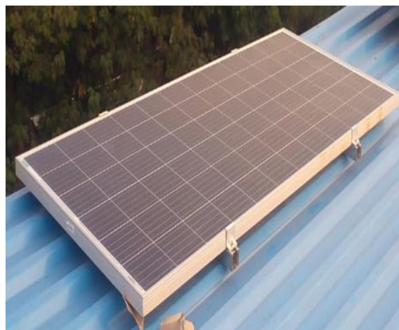
390 Watt Solar Panel Mounted on College Terraces
