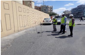
Figure 4: Fault pin-pointing for fault under asphalt
