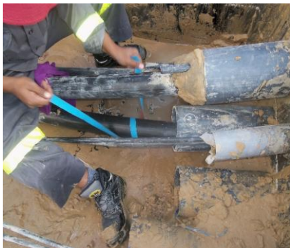
Figure 5: Fault inside road crossing duct rectification
