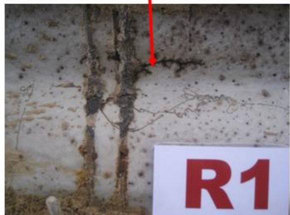
Figure 3: Sample of fault over joint
