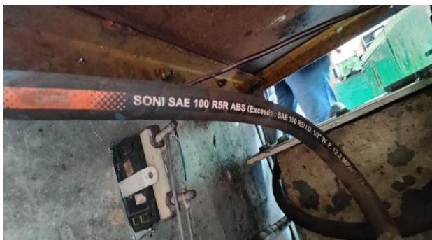
Figure 3.8: Hydraulic hose pipe
