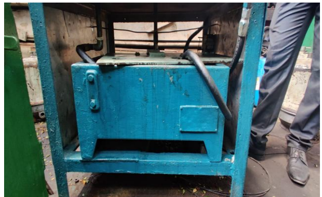
Figure 2.9: Lube Oil Tank
