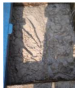
Figure 2: Sludge tank before Bioaugmentation
