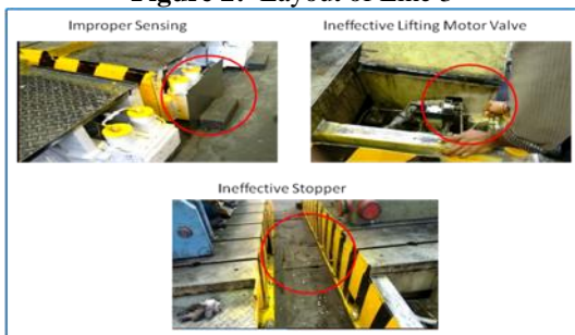
Figure 3: Improper sensing, ineffective method of lifting the motor valve, ineffective stopper
