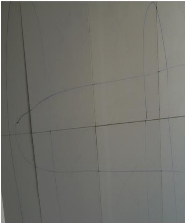
Figure 5: Swelling of plaster and tiles in third floor bathroom
