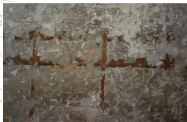
Figure 2: Corrosion in RCC due to insufficient cover
