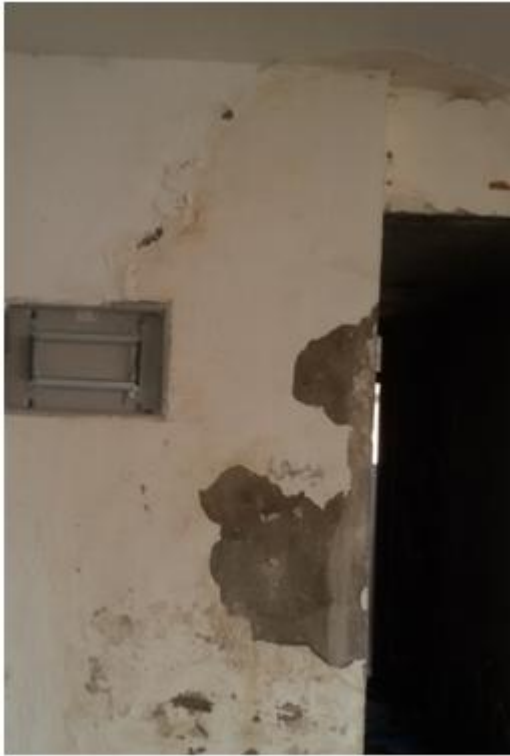
Figure 4: Dampness in wall adjacent to bathroom
