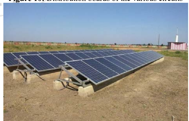
Figure 11: The photovoltaic system and the VOR station.
