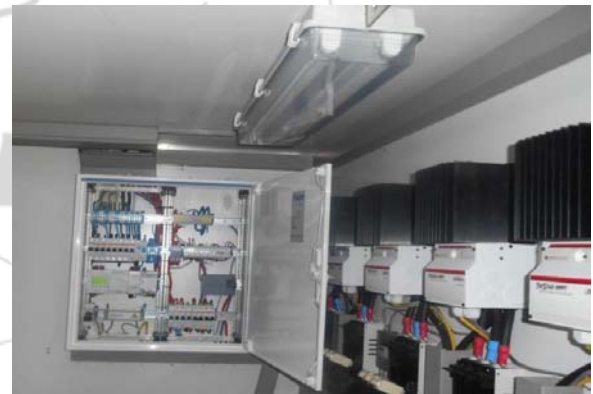
Figure 10: Distribution boards of the various circuits
