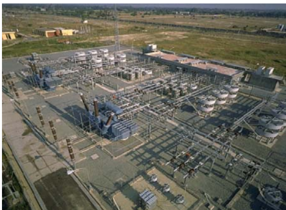
Figure 7: SVC installation model- source: Siemens
